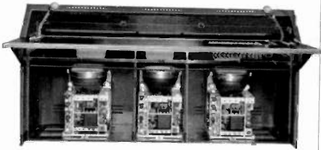
TC-5A front cover removed to show mounting of monitors
