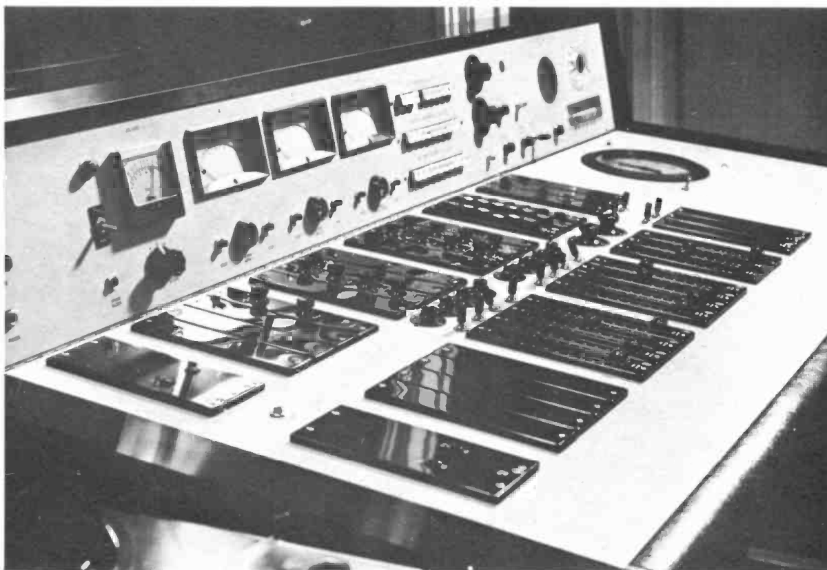
Recording Studio Console at Dick Charles Recording Service, New York City designed by Gotham Audio Corporation; built by Magna-Tech Electronics, N.Y.C.
