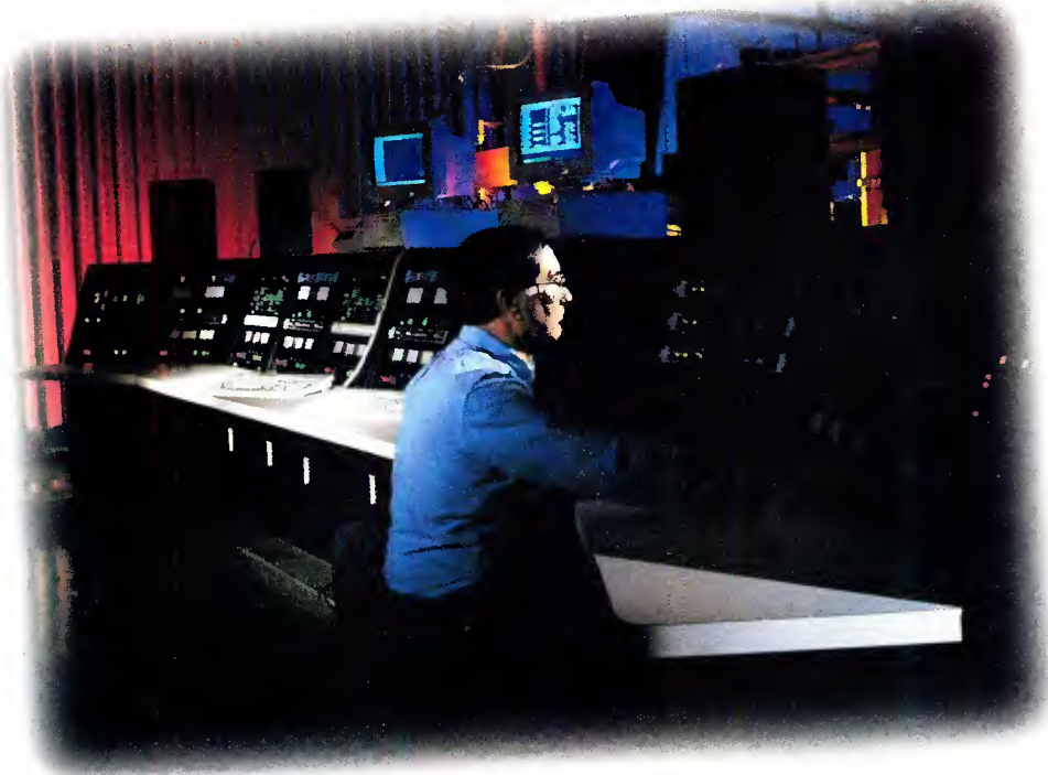
Control console for 120 kW FM system
