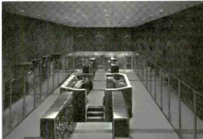
VOICE OF AMERICA —Six Gates 50,000 watt Model HF-50C transmitters in use at the Greenville, N. C. transmitting station.
