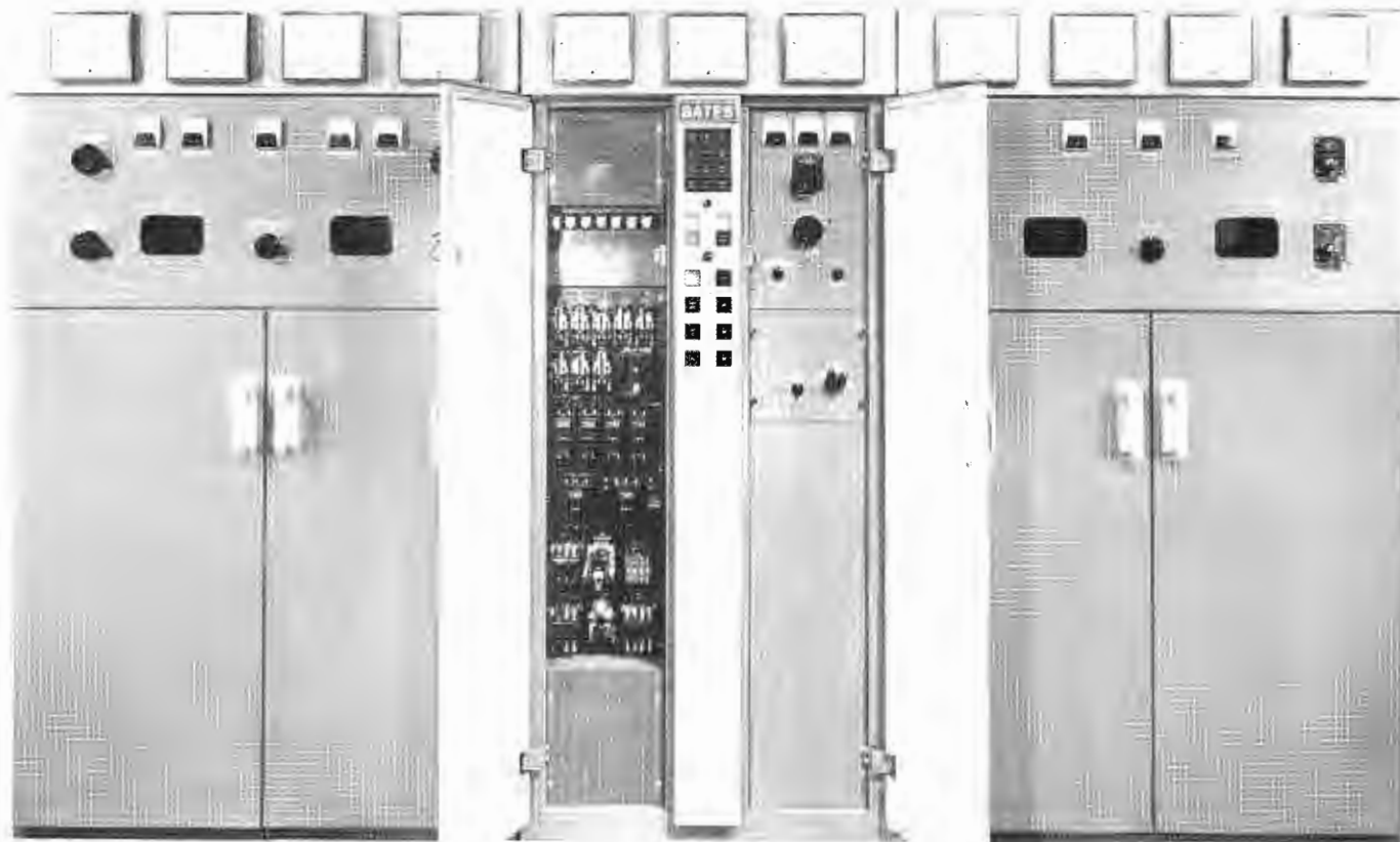
Front view showing supervisory and exciter cubicle.
