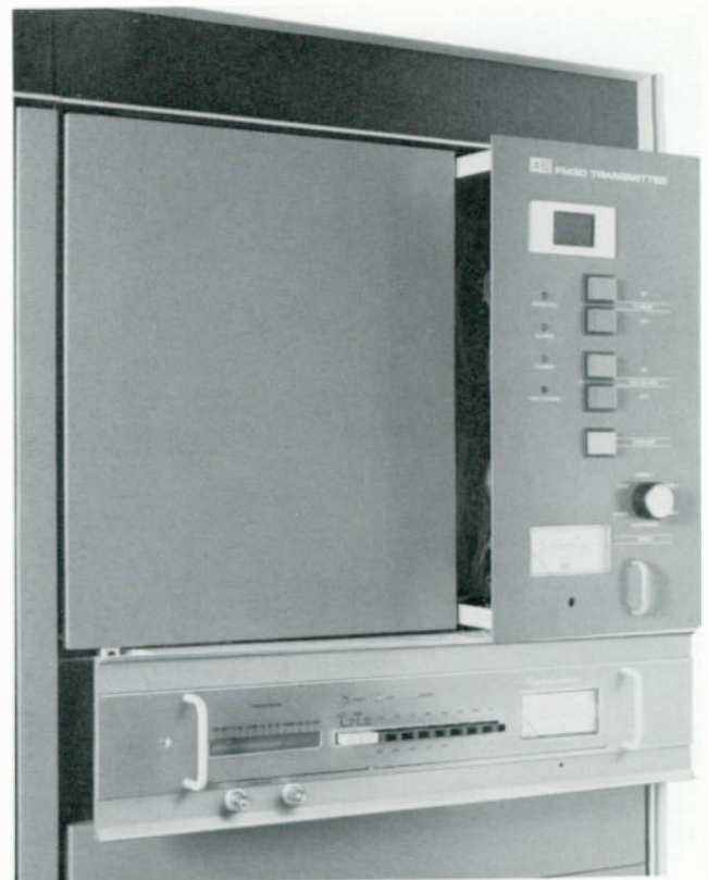
All transmitter control and status functions in the FM-30 transmitter are performed by a built-in microprocessor controller (upper right part of photo). The advanced design Model FX-30 exciter is in the lower portion of the photo. Both units slide out for easy access.
