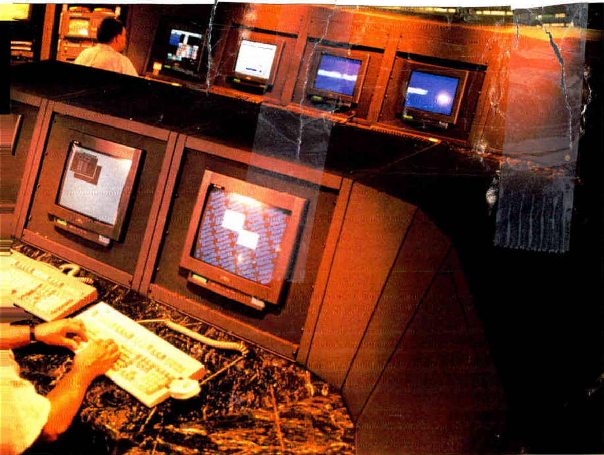
Jones Communications' headend facility in Alexandria, Va. is considered by many to be state-of-the-art.
