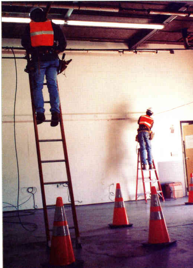
Two trainees practice installing aerial drops at RTK's Northeast Region Training Center.
