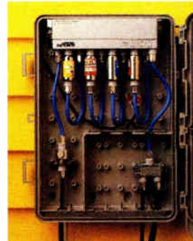
Fully-configured STARPORT unit within an on-premises enclosure.
