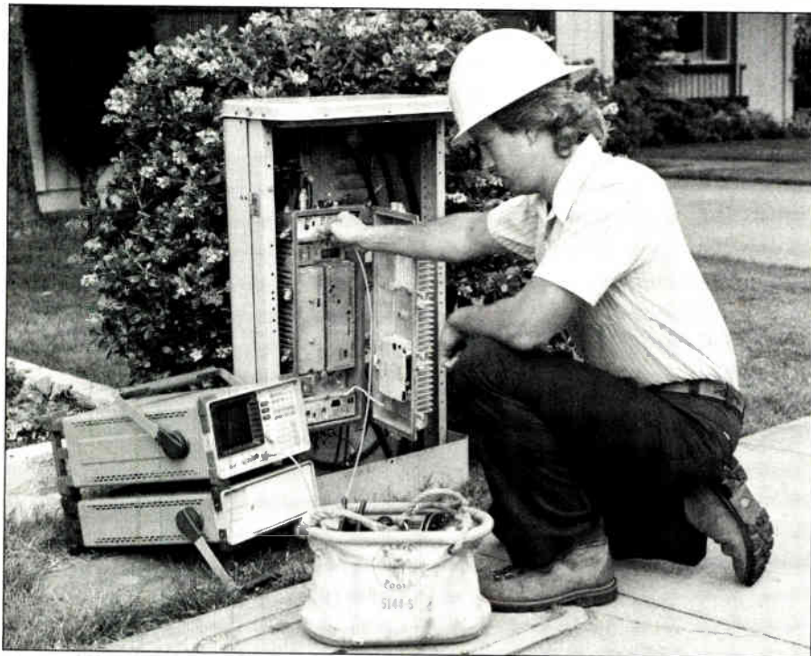
A portable spectrum analyzer performs CATV tests at the cable terminal box. A portable AC power source provides power for field operations.
