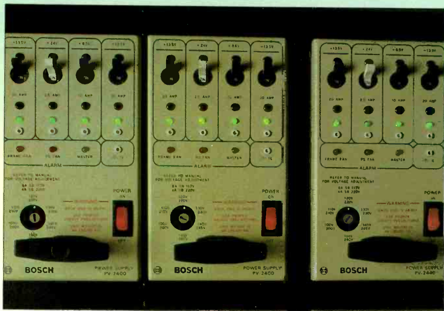
These BTS power supplies provide the power to activate the BTS routing switcher.
