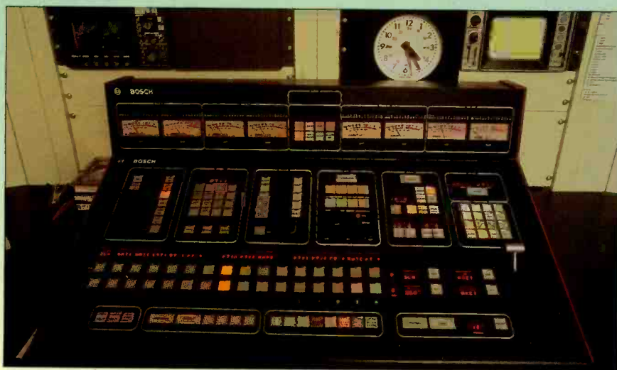
Opening page: Engineer Ken Corcoran in the channel 44 master control room with his hand on the microwave switcher. Like much of the new equipment, the switcher is an in-house product. Above: BTS model 2000 master control switcher located in the channel 2 master control room.
