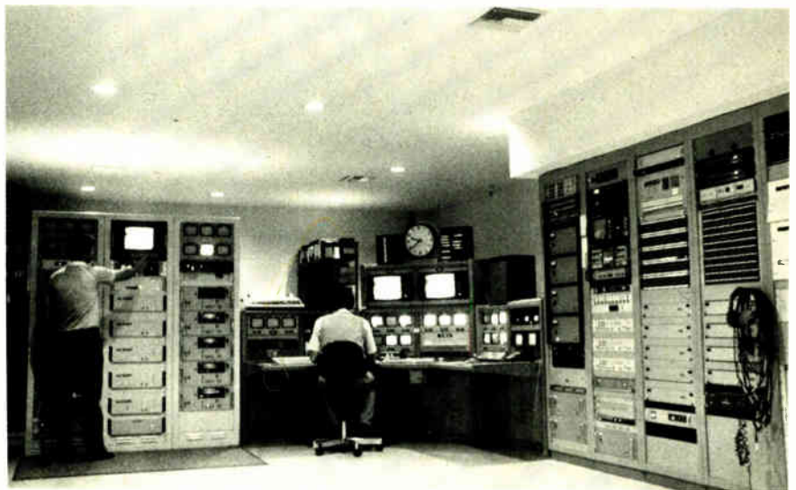
Master control includes the Lake Systems La-Kart II system, the key to KSCH's automation.
