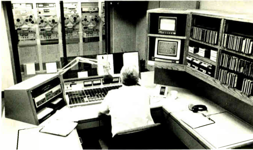
Announcer Bill Norris is able to look into the room, which holds equipment racks from KQXT-FM's on-air studio.
