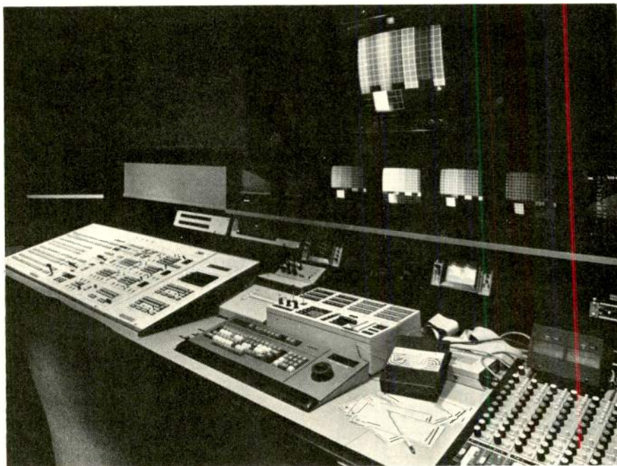
Edit Room 3 at Broadway Video. Interfaced through the BVE-5000 editor are a CD-480-10 switcher with CAP, the Mirage 3D effects system, a Thomson-CSF Vidifont Graphics V, and a Soundcraft audio board.
