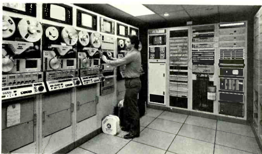
Broadway's Chief Engineer Martin Zofcin adjusts VTRs in master control area, completely invisible to clients.
