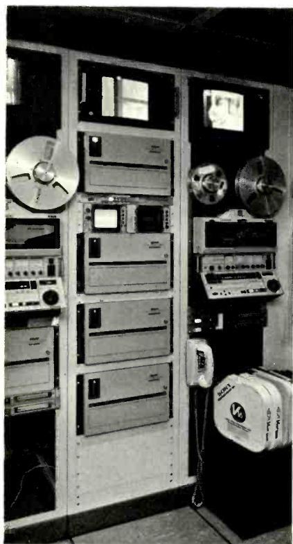
Four Sony BVH-2000 VTRs are assigned to Edit Room 3 and can be patched together with additional decks if required.
