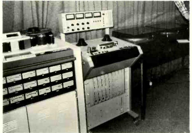
ITC carts, Yamaha console, auto-locators, and nearby patch panel viewed from engineering position.
