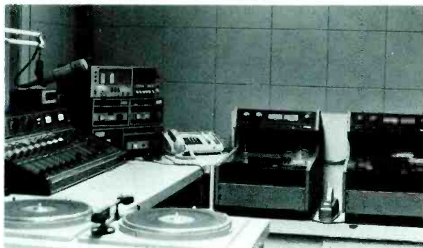
Studio C is normally used for production, but can be used on either AM or FM with such equipment as the BE console, Otari reel-to-reels, ITC cart decks and JVC cassette.
