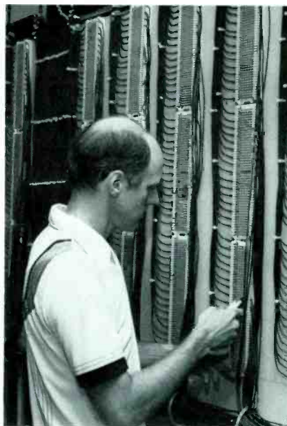
Engineer John Morton works on interconnect system on wall running in back of operations area. All leads from racks come to jack fields on wall; all interconnections are made there at normal working height.
