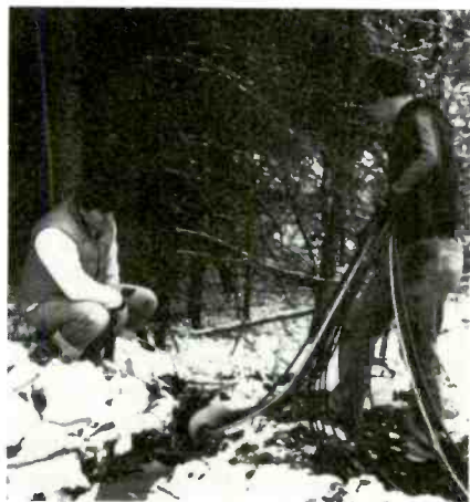
Workers install cables in underground conduit. Light-colored cable is Galite Company's six-cable fiber optic link between broadcast center and Opening/Closing Ceremony venue
