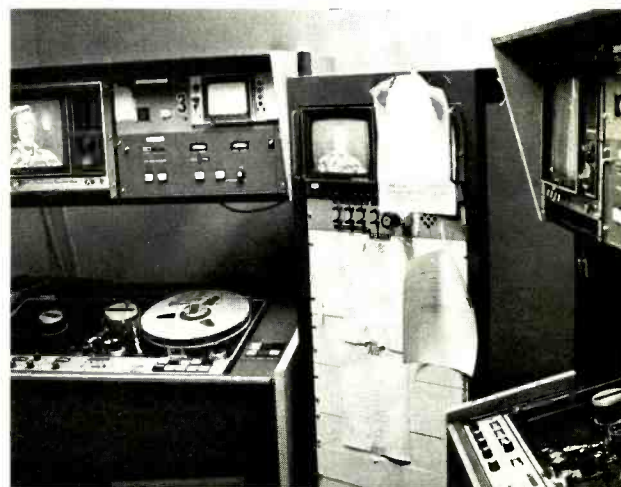
CITY is unusual in that the principal on-air equipment consists of IVC-960's. These units, in production room, are equipped with editors. Ampex's Model 800 TBC is used.
