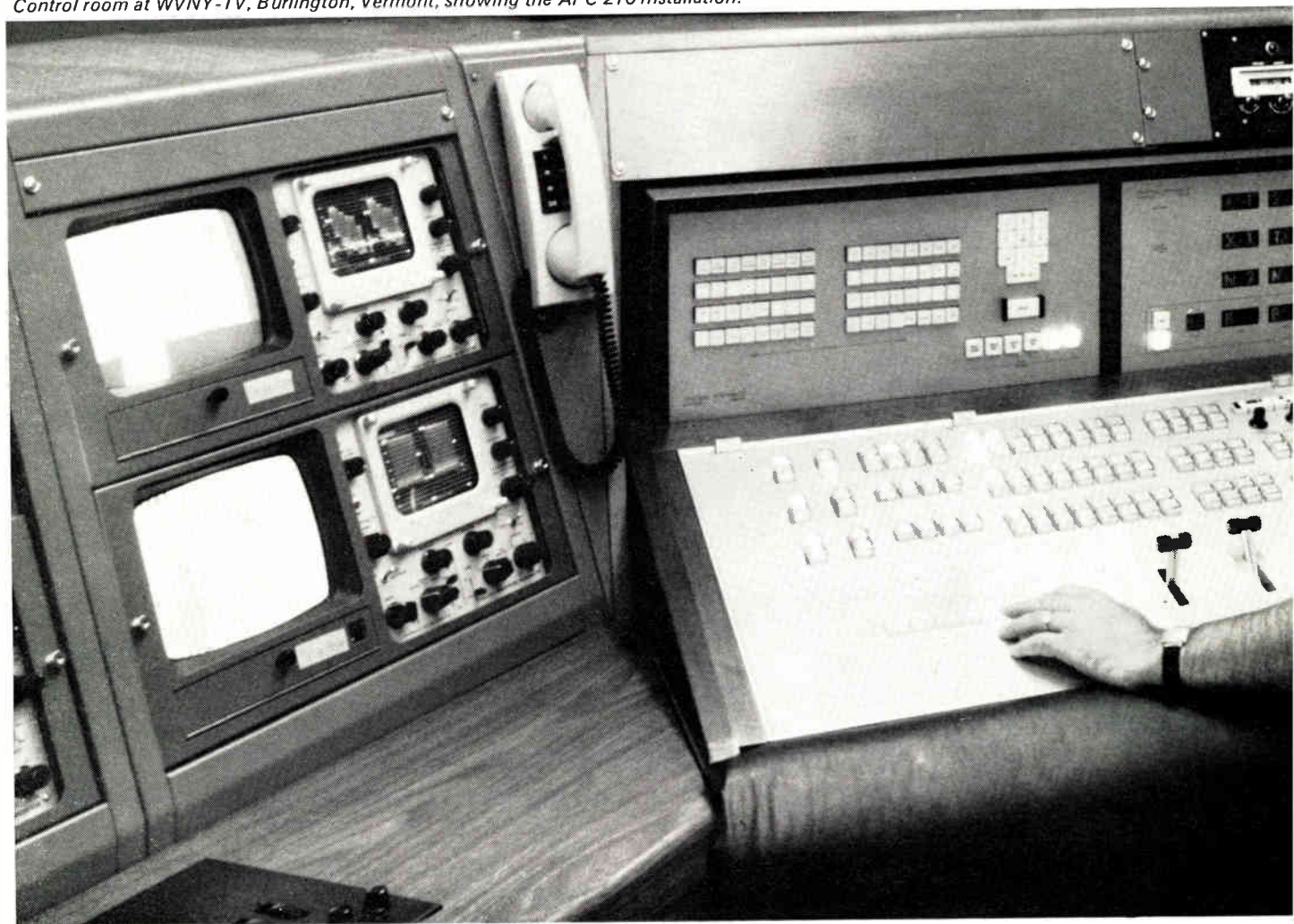
Control room at WVNY-TV, Burlington, Vermont, showing the APC 210 installation.
