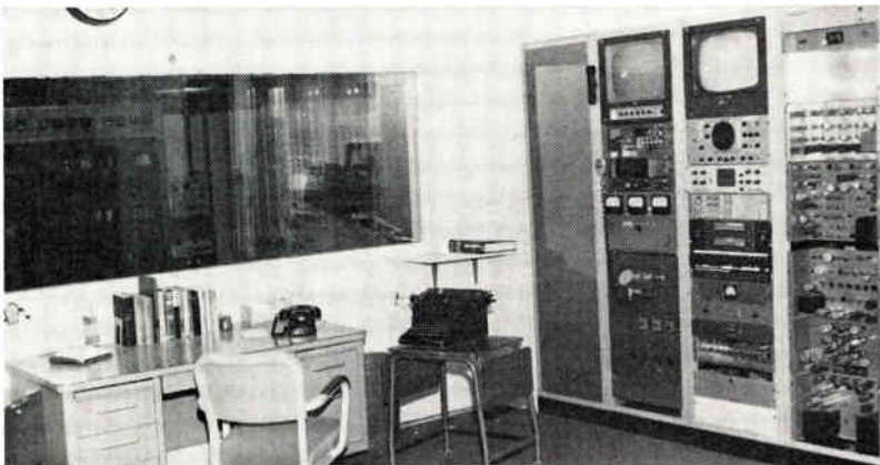
Control room installation for transmitter.
