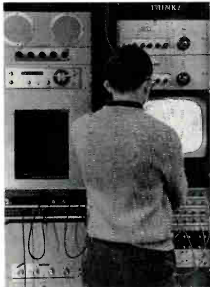
CCTV distribution panel at GVSC
