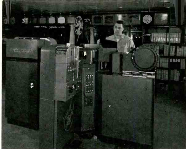
Color film chain installation at KSTP Minneapolis includes two 16mm and slide projector, colorplexer, and camera.
