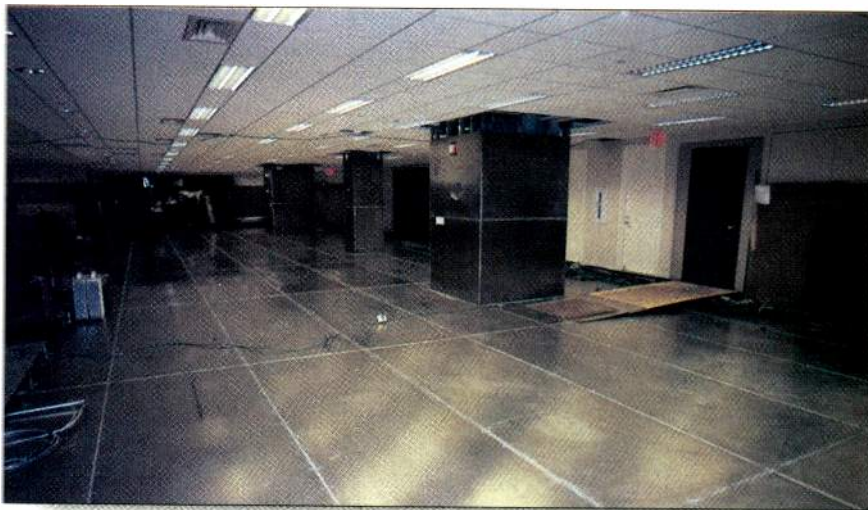
The installation of shielding is often required to reduce elevated magnetic field levels in areas containing sensitive equipment. Photo courtesy Field Management Services.
