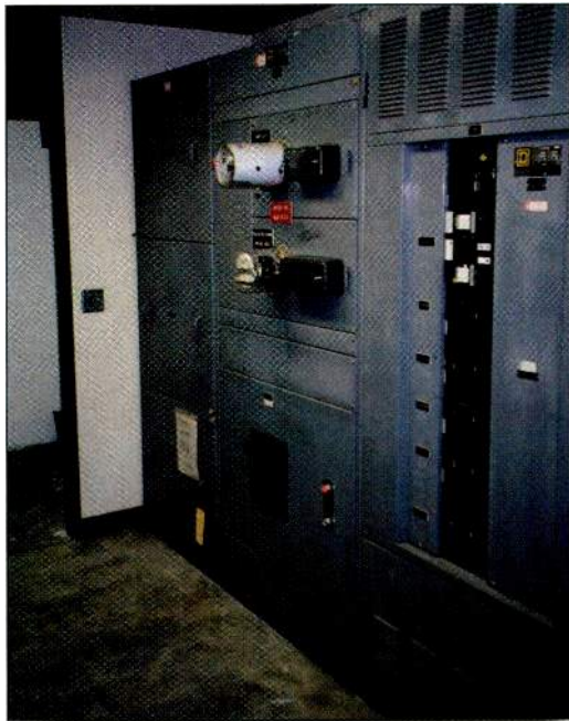
High-current electrical components such as transformers and distribution equipment generate large magnetic fields in adjacent areas. Photo courtesy Field Management Services.
