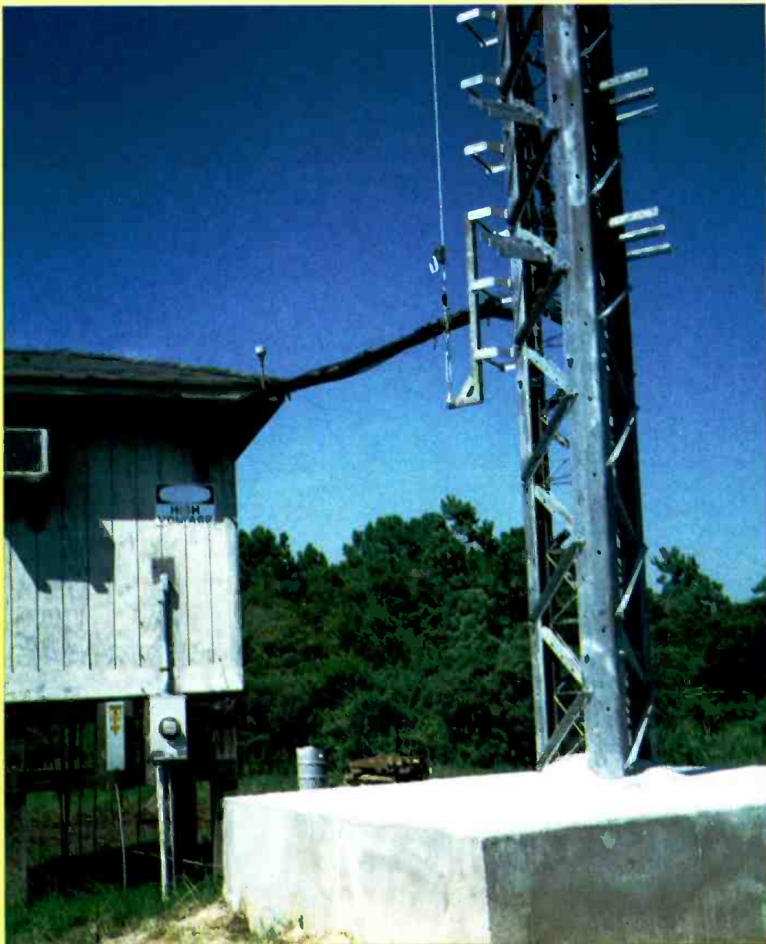
The base portion of a small 18-inch face tower on which the augmentation process has been completed. The new larger augmented foundation is an indication of the load this tower is now prepared to carry. Also shown is the coaxial cable mounting members extending outward from the tower face. (See Figure 2.)
