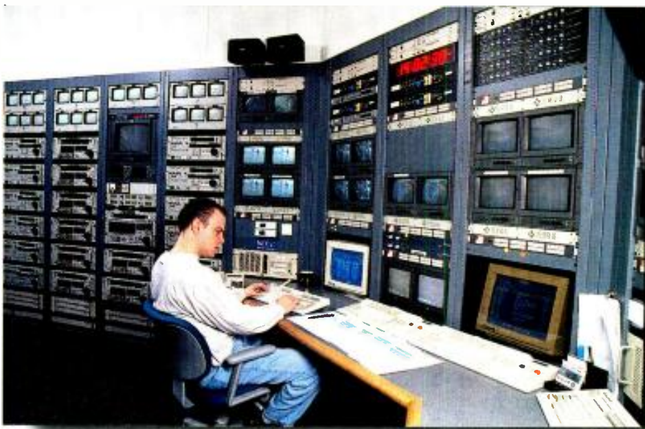
Master control room for request pay-per-view movies. This room runs five channels, sending feeds in both C-band and Ku-band for uplinking.
