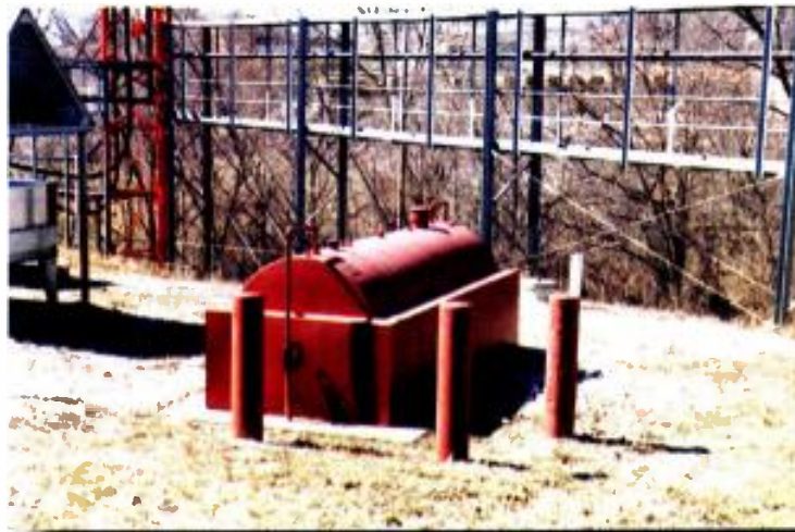
Local regulations vary regarding fuel tank installations. Check with the authorities and your insurance carrier to be sure you comply with all applicable rules and regulations.
