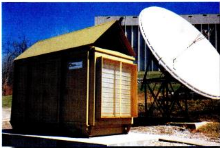
Standby generators can be reasonably self-contained, but require a stable mounting surface and considerable airflow.
