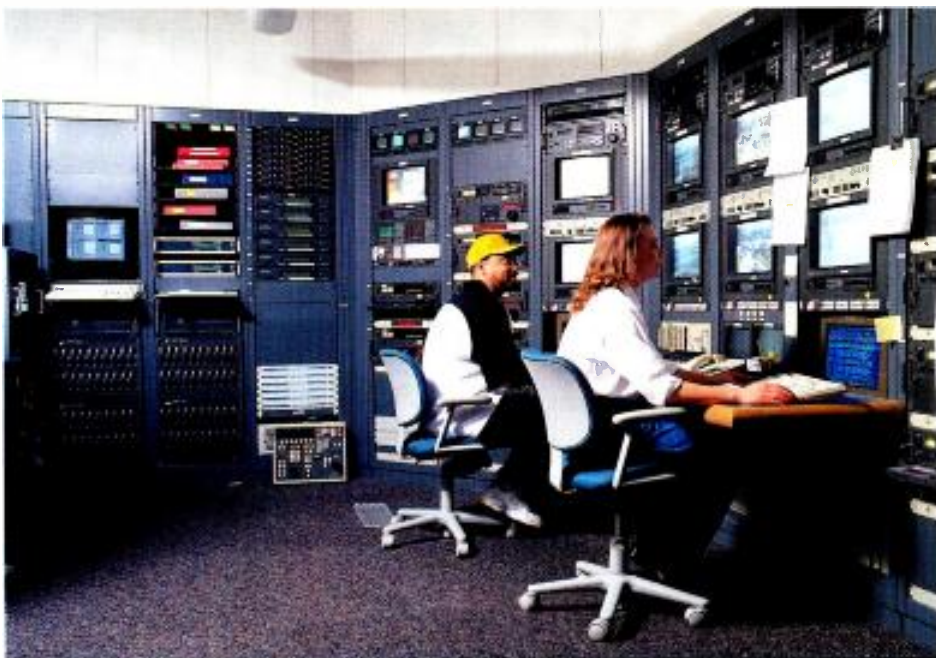
Eight-channel control room for Your Choice TV. Note servers in left background.
