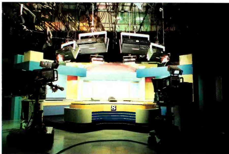
The Videssence lighting system in use at the news studio at KGW Northwest NewsChannel 8, in Portland, OR.
