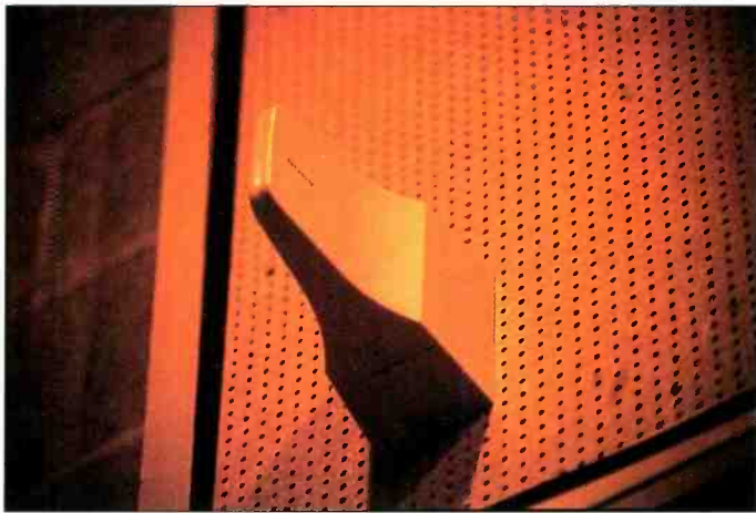
One of a pair of diversity receive antennas for a permanently installed UHF wireless microphone system. The other antenna is mounted on the same studio wall, about 30 feet away.
