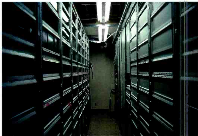
This large-facility, 300x320 analog-crosspoint intercom matrix occupies 16 full racks. Rectangular matrices such as this must grow in proportion to the square of the number of users. A new digital intercom system could reduce the size of this matrix to a single rack. (Photo courtesy of ABC Broadcast Operations & Engineering.)
