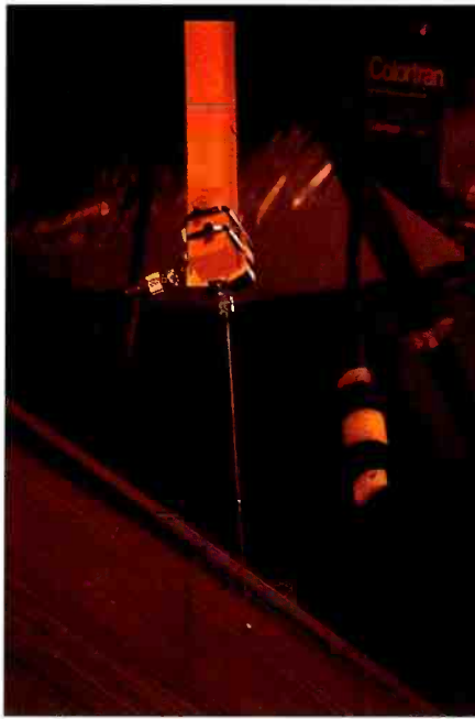
A VHF wireless mic receive antenna at WXIA-TV, Atlanta. The antenna is mounted on a non-RF-reflective pole hung from the ceiling above the news set.
