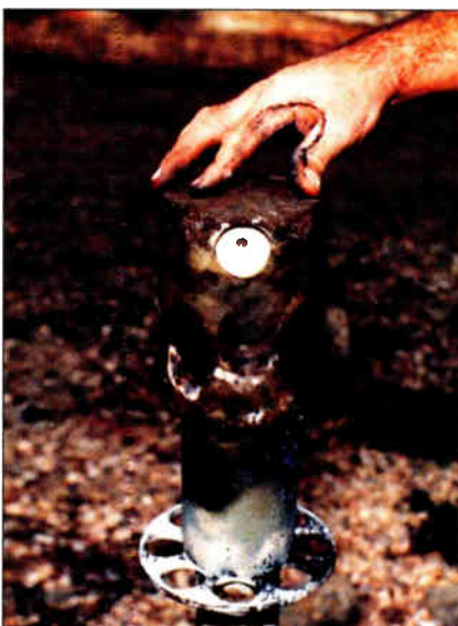
Dust-laden moisture forms a conductive path, as indicated by the burned Teflon. As the path arcs over, transmission line failure occurs.
