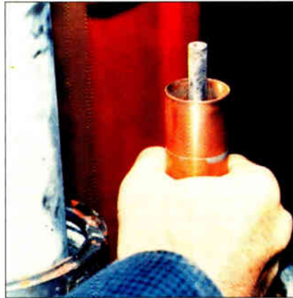
Moisture in a transmission line can result in corrosion that increases attenuation and degrades system performance.
