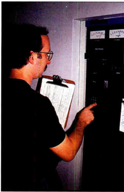
To avoid major failures occurring when no technical staff is on site, the contract engineer must watch for troublesome trends at each visit.
