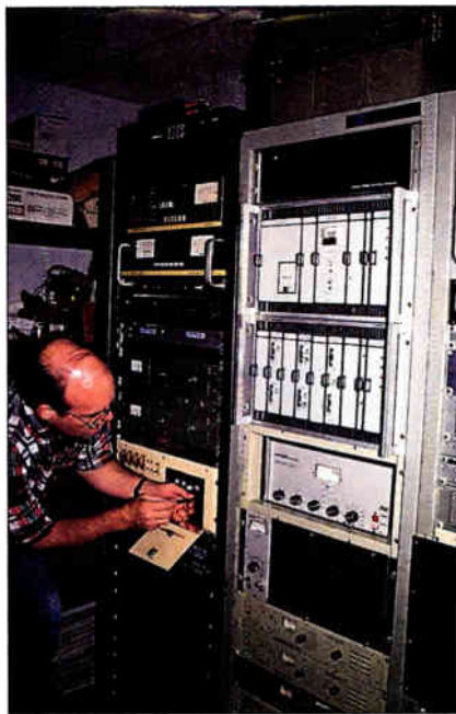
Taking pride in the quality of the air signal is an attitude that contractors should adopt for every station they service.
