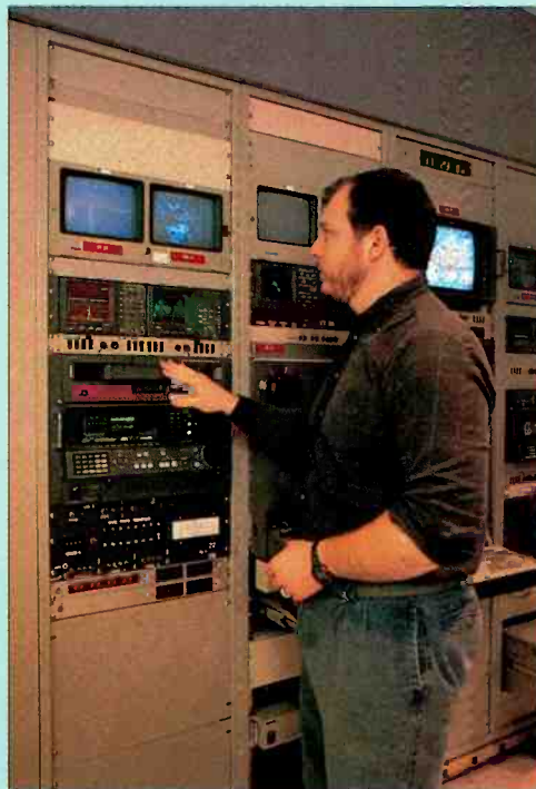
The dub/verify QC station in use at TBS. The time-code encoder is located above the tape machine, the custom 2-rack unit is below the tape machine.
