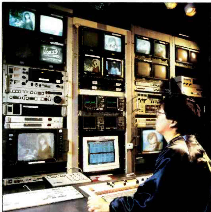
KHNL/KFVE master control, showing automation terminal display on monitor at bottom of center rack. Note dedicated control panel for automation system on counter behind QWERTY keyboard and switcher.
