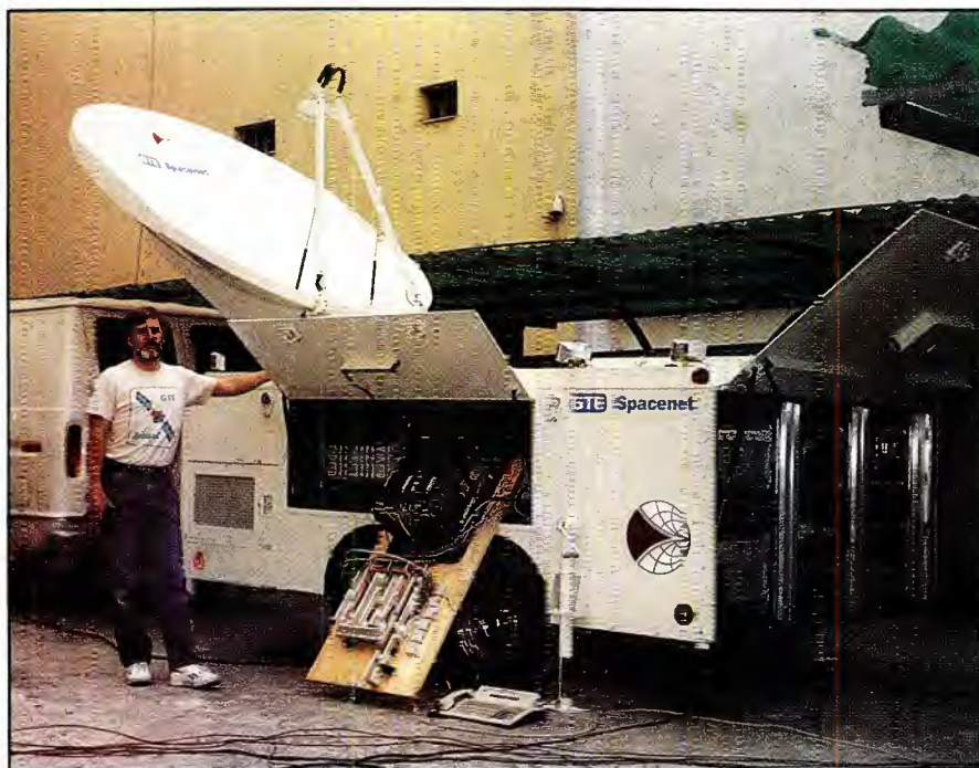
Despite a tangle of red tape, the remote crew took this demand assignment multiple access (DAMA) satellite communications system to Cuba for coverage of the ill-fated Reagan-Gorbachev meeting.
