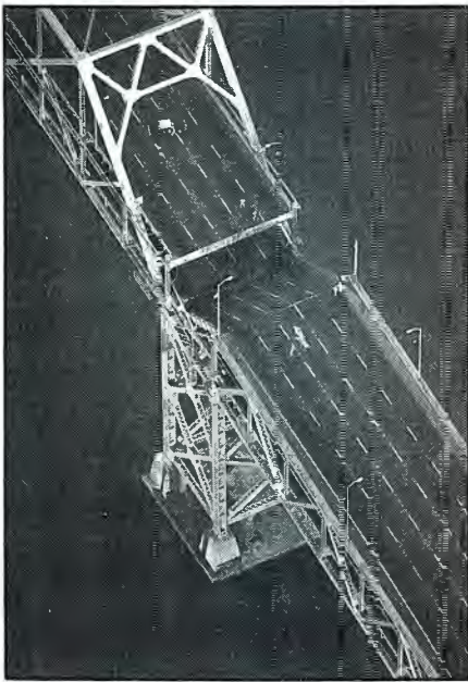
The importance of building high-rise and high-weight structures on bedrock was emphasized by the failure of a portion of the Bay Bridge, which runs between San Francisco and Oakland. The concrete pier moved during the quake, pulling the bridge apart like a toy. (Photo by Deanne Fitzmaurice, San Francisco Chronicle.)
