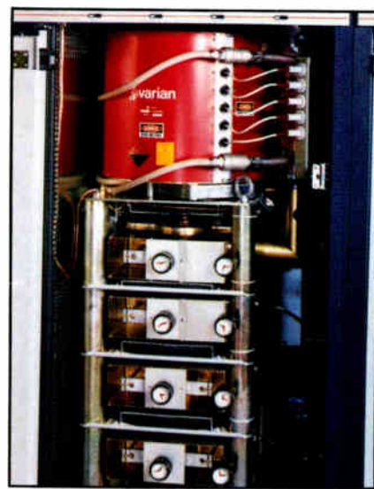
MSDC klystron mounted in a 60kW transmitter. The tube is identical to a conventional klystron except for the collector assembly.
