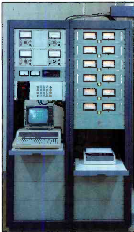
Accurate and complete monitoring is essential to a reliable multiplexer system. The arrangement shown features continuous monitoring of forward and reflected power for each of the six stations using the multiplexer. A computer processes electrical and environmental data to manage site operations.
