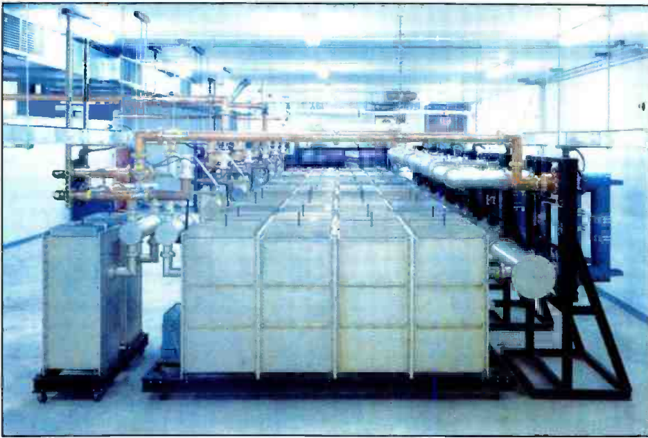
Large multiplexer systems require a great deal of floor space. Depending on the number of stations to be combined, the multiplexer may be configured to fit the physical space available. Note the use of casters on the individual modules of this combiner to make installation easier.
