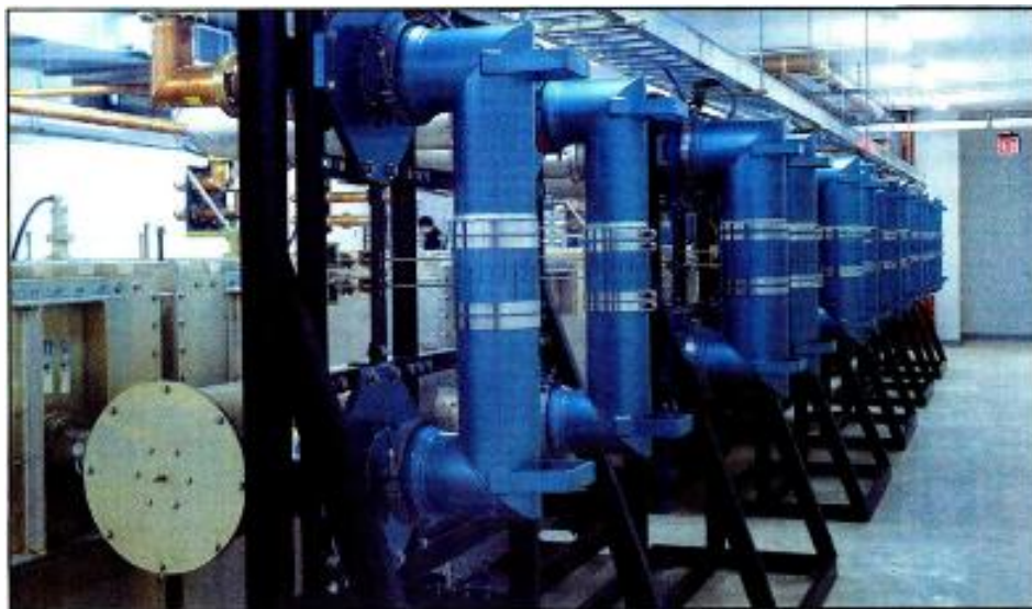
Multistation FM combiners have gained considerable interest since the FCC's 80-90 decision. Systems can be large or small, but the idea is always the same: Feed two or more transmitters into a single wideband antenna.
