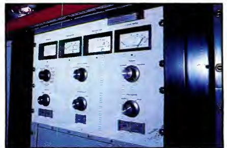
The front panel of the transmitter can tell a great deal about what is going on inside. Make a complete check of all operating parameters on a regular basis.
