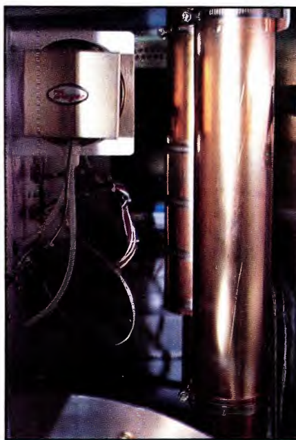
Check transmission line hardware for overheating and mechanical tightness.
