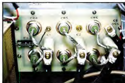
Check the heating of individual rectifiers in a stack assembly. All devices should generate approximately the same amount of heat.
