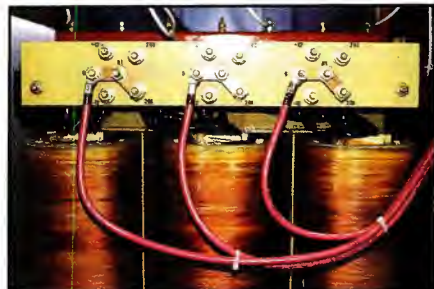
Inspect power transformers just after sign-off for indications of overheating or leakage (in the case of oil-filled transformers).
