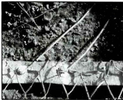
These two radials were connected to the ground screen with rivets. After a few years, they failed to provide an adequate connection.
