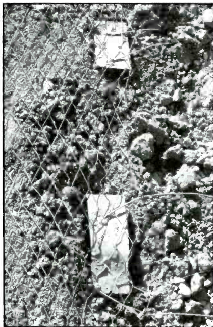
Small pieces of copper strap were used to attach the radials. It is far better to use a solid piece of strap around the perimeter of the ground screen for these connections.
