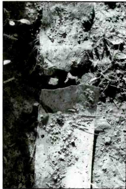
Even though the copper strap may appear undamaged, give it a strong pull. This strap came apart with little strain.
