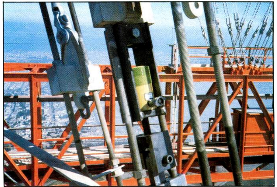
Guy tension for the antenna stacks. Note the hydraulic ram in the center. The RF-protected sixth-level riggers' shack can be seen at the far right.
