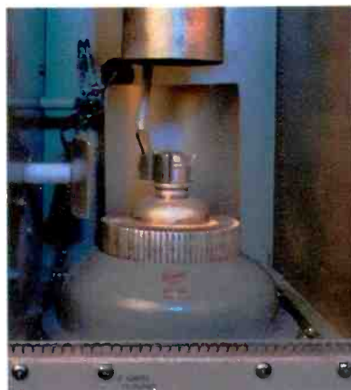
EIMAC's 5CX1500B broadcasting tube in KGLT radio station's transmitter.
