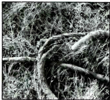
This romex cable was buried without conduit protection.
