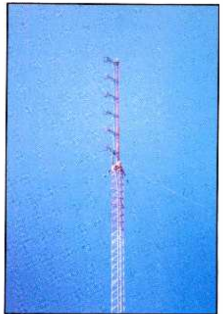
The top section of the 660-foot tower after the FM antenna was mounted.
