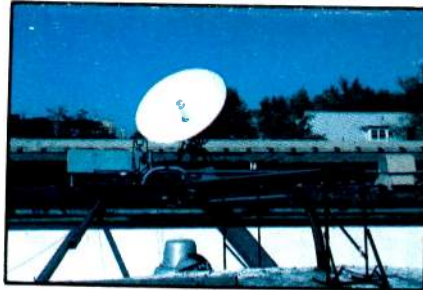
NNS downlink TVRO is situated on the TV station studio roof and is less prone to vandalism. An ice-bridge protects the feedline from falling ice off a nearby transmission tower.
