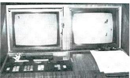
Close-up of studio floor terminal.
