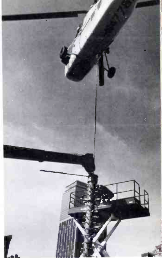
Spiral antenna bay is tilted vertical and technician attaches cable to hovering helicopter.
