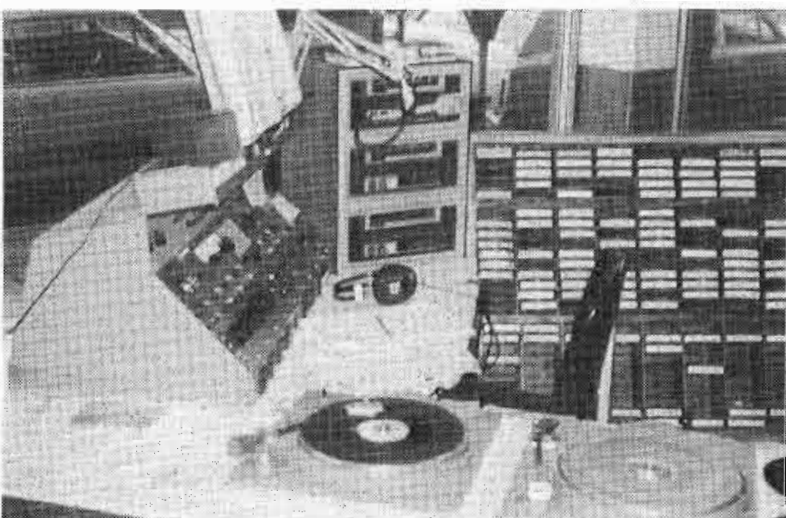
Fig. 4 KISN uses a streetside studio. The station uses a digital timer which resets each time a function is initiated via a momentary closure/pulse. This is useful in maintaining a tight program format.
