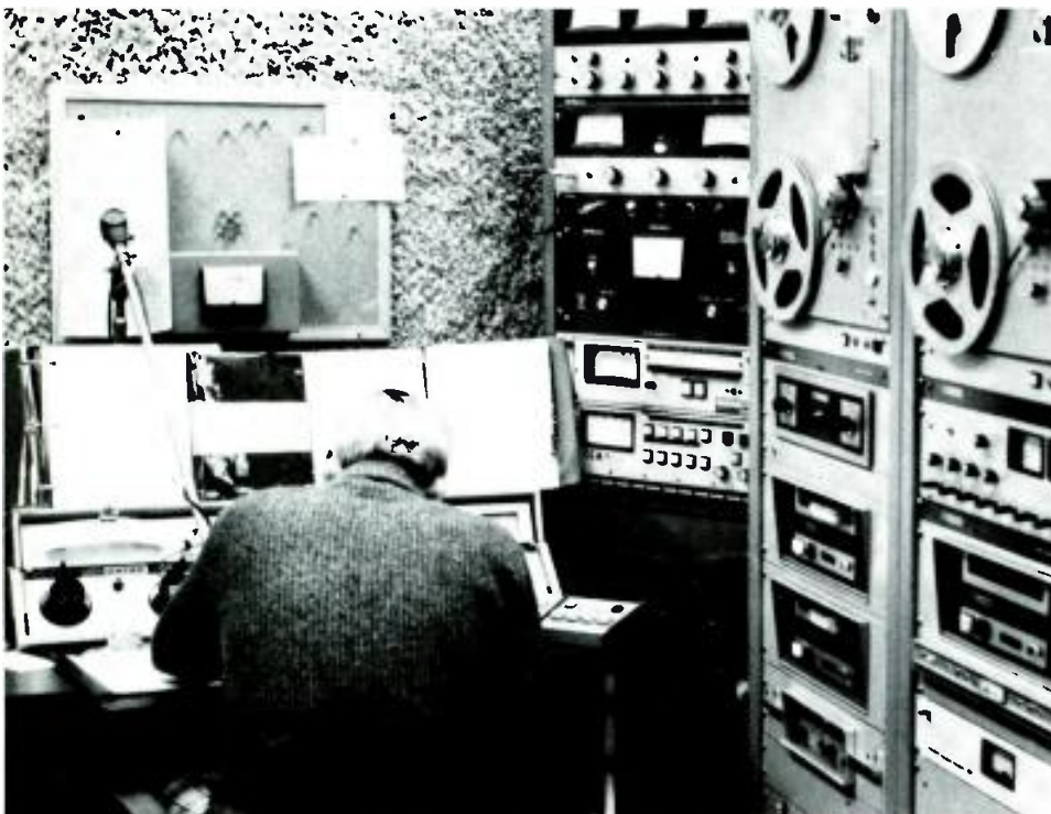
Inside the WLAK control room where automation sound is optimized. And it doesn't hurt to carpet the walls!
