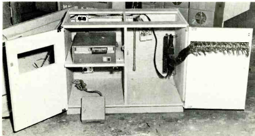
Fig. 4 When desk panels are open, there is easy access to all cables.
