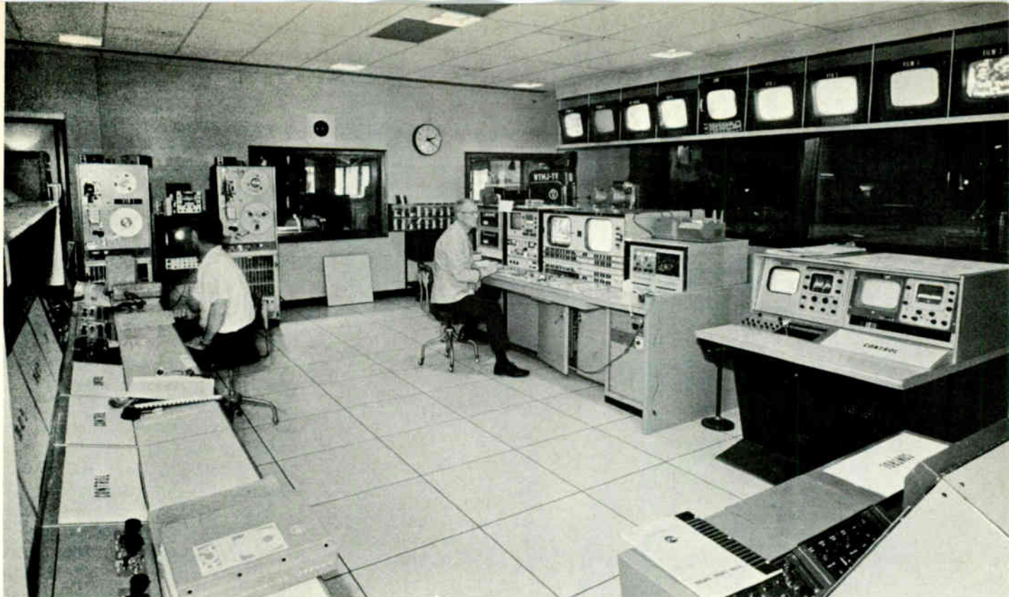
WTMJ central control room.
