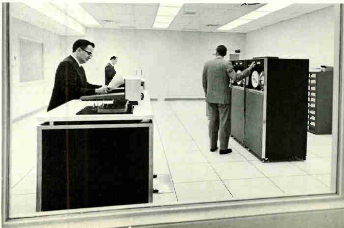
Hallway view of computer complex.
