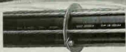
870-foot self-supporting catenary installation of 5 inch HELIAX air dielectric coaxial cable (Type HJ9-50) at mountain top site of Station KBYU-TV, Provo, Utah.
