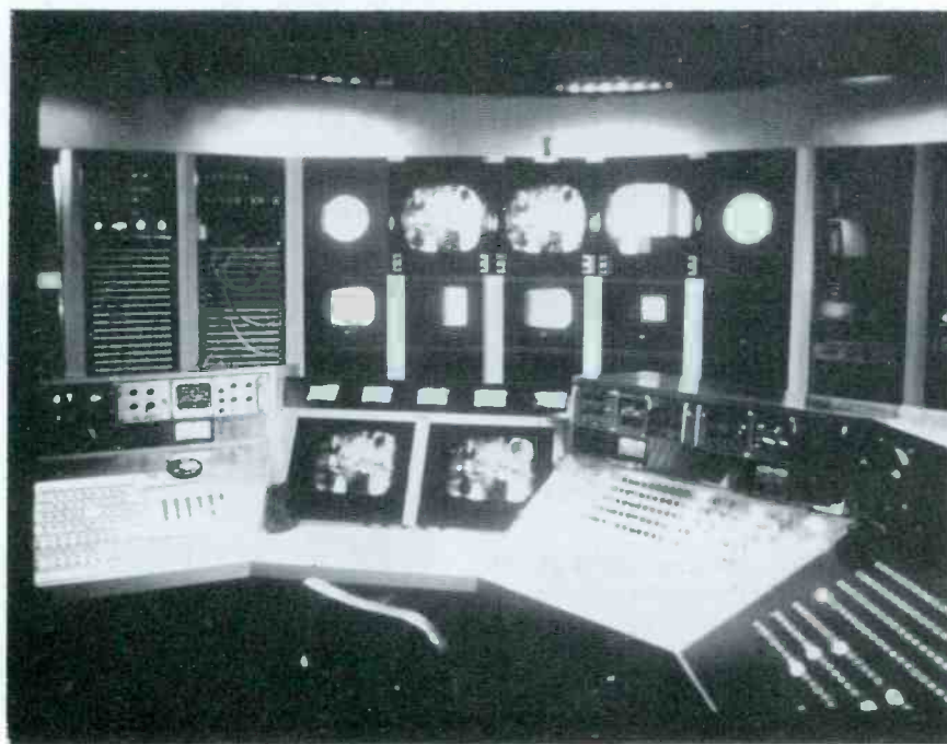
Radio and television master-control operating desk for the entire center.
