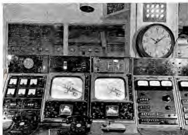
Fig. 2. CFCF section of the desk with all monitors and metering.
