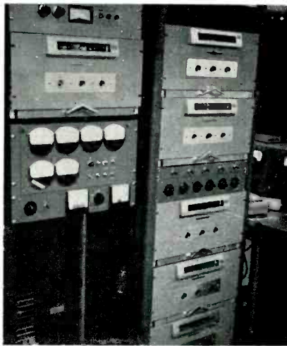
Fig. 1. Radio control room equipment.
