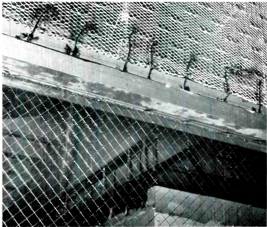
View of wall between receiver room and control room of the receiving center. Note wires welded to metal lath for electrical bonding and grounding. Similar wires, visible at top of wire glass, will be used to electrically bond and ground the wire mesh within the glass. For shielding purposes, all metal within the receiving center and two transmitter stations was bonded and grounded at four-foot intervals.
