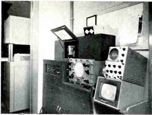
Figure 2. The weather radar pickup system at WDSU-TV New Orleans.
