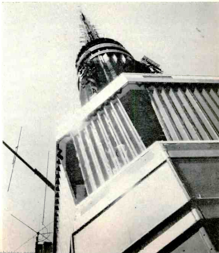
Figure 5—Skyward shot taken from the observation deck of the Empire State Building shows the final installation work on one corner of the east side enclosure.
