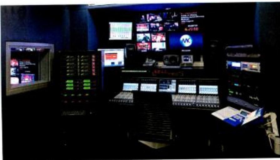
Adjacent to the control room is the audio mixing suite. The overall communications system is based on a Riedel 136 x 136 matrix with a combination of analog, MADI, and AES and GPI interface cards.
