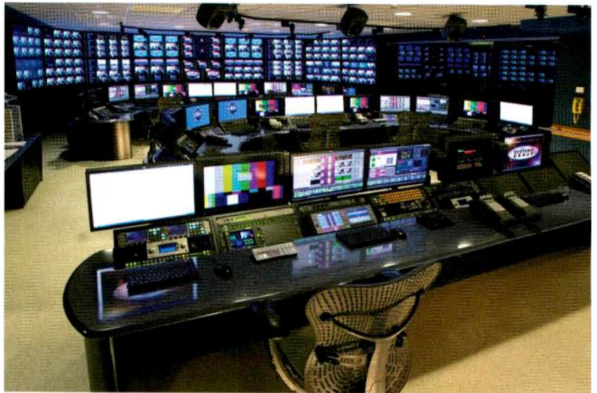
One of the interesting aspects of ABC Television’s new central routing and switching system is that it incorporates technology from a number of vendors.
