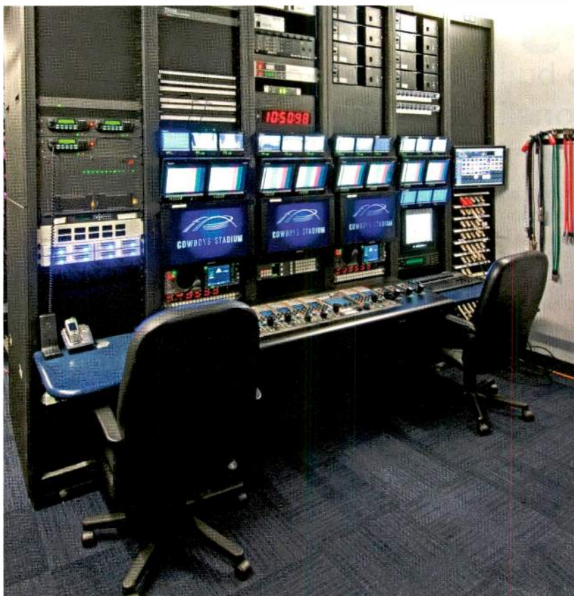
This control room employs dual camera shading positions for 16 stadium cameras, a Riedel Artist intercom and triax patch panels.
