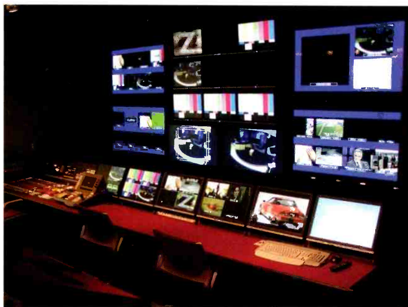
The WFYI facility features two control rooms, which can be operated individually or in tandem for larger productions.
