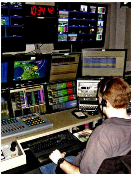
Control room automation at WFTV, the Cox Media Group station in Orlando, FL, is helping the station realize greater staffing efficiencies and produce tighter newscasts.
