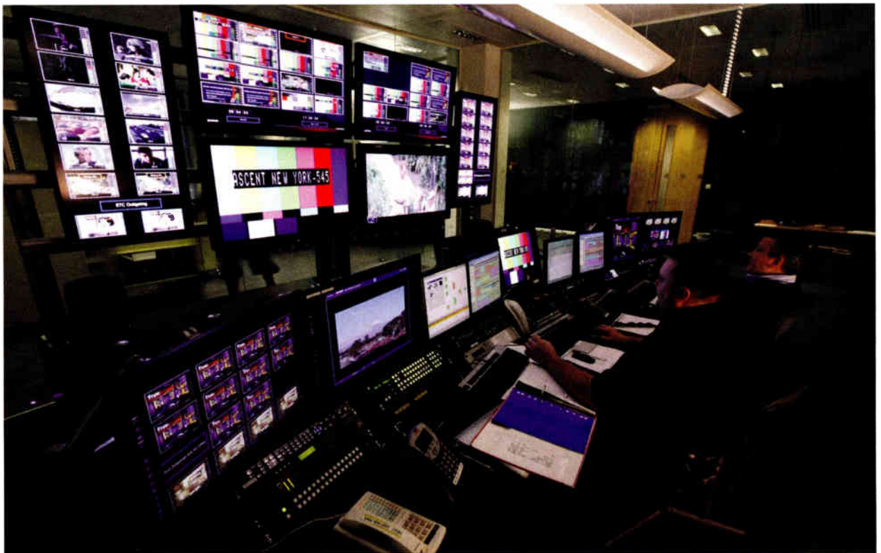
Ascent Media is an example of a broadcast/production facility that has integrated the multiviewer element within the core house routing system.
