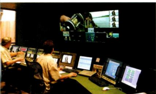
The Outdoor Channel's control center features a DVEO T-Streamer, which is fed by an ATSC-compatible stream from a DVEO QuadMux.
