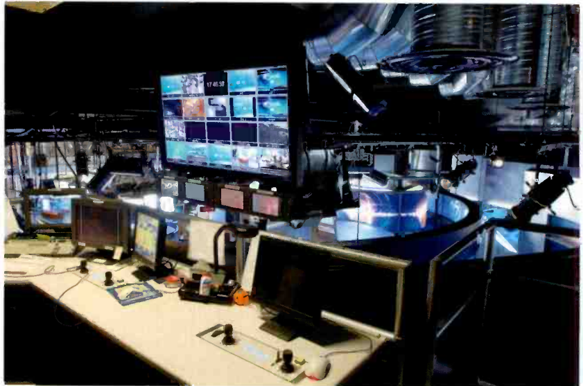
The robotic operator position consists of two Vinten camera and robotic control positions for redundancy. The Vinten controls can be operated by the touch screen or mouse.
